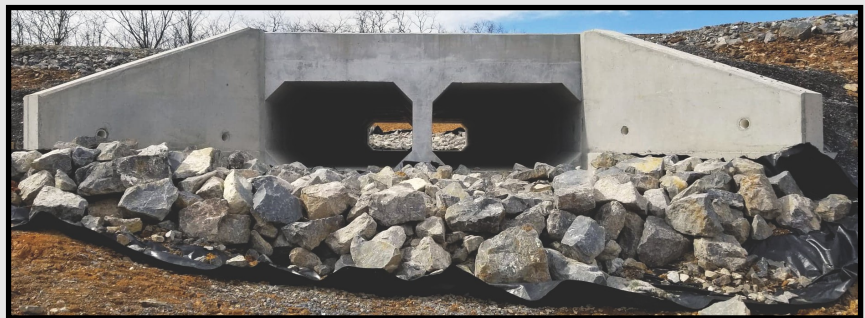
Above photos: side view, finished double box culvert with wing walls completed mid-March 2020 in Winchester, VA
